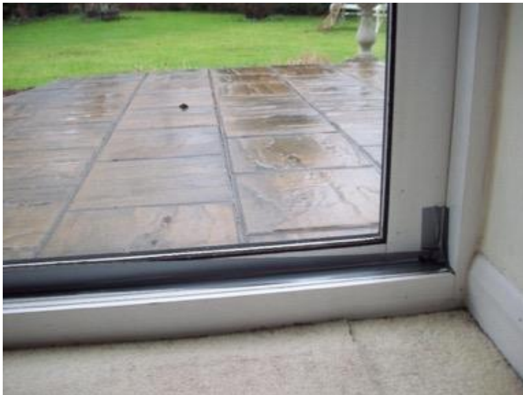
Patio door still taped up after flood water had retreated
