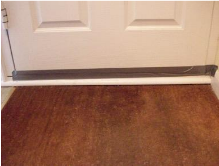
Inside front door – taped
